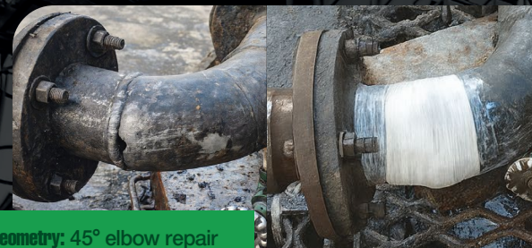
Leak Sealing: Application of MaxeWrap to a water line with an active leak.
